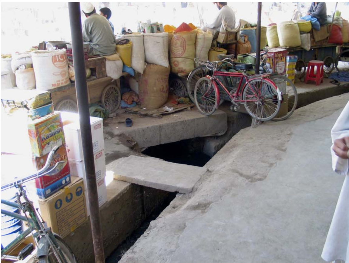
A market scene showing some hazards caused by having open trenches in congested areas.
